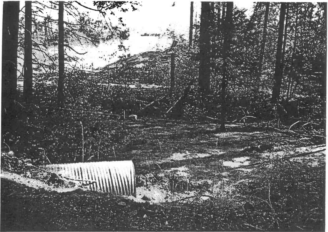
The culvert at site 80F-1 suffers from considerable accumulations of fine sediment delivered from over 1000' of entrenched roadway.
