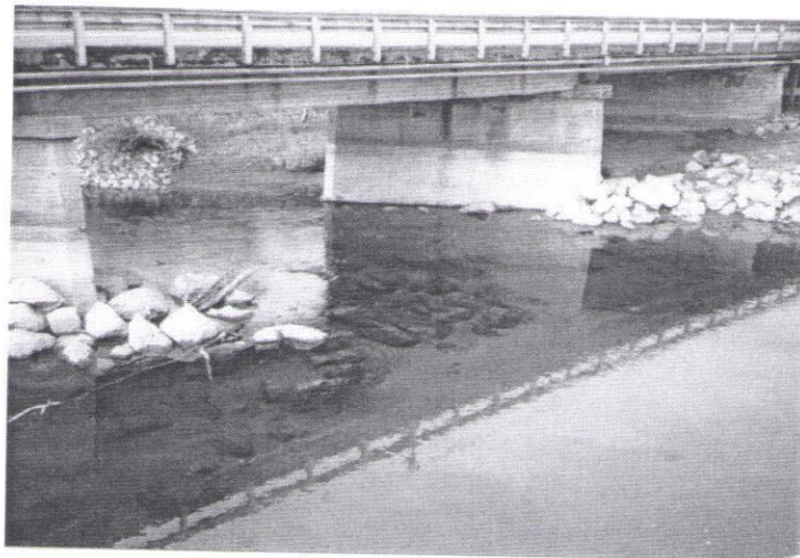
Figure 3-14: Large rip-rap placed around piers under the Midway Bridge after the January 1997 high flow to control scour. (The light surface in the lower right corner is the reflection of the sky.)
