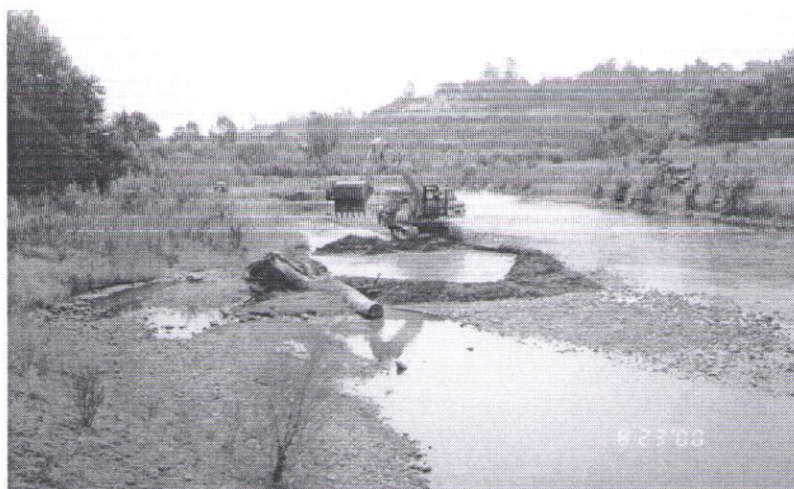
Figure 5-2: Equipment removing gravel from the channel upstream from the Parrott-Phelan Dam to maintain channel capacity.
